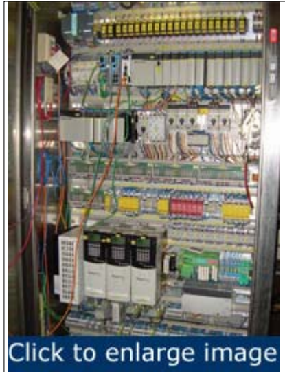
Figure 1. This automation cabinet contains power, control, and communication wiring. A 480-V disconnect handle is at the upper right of the cabinet. PLCs near the top of the cabinet use 24-V inputs and outputs to control a conveyor system while 480-V VFDs near the cabinet bottom drive the conveyor motors.
